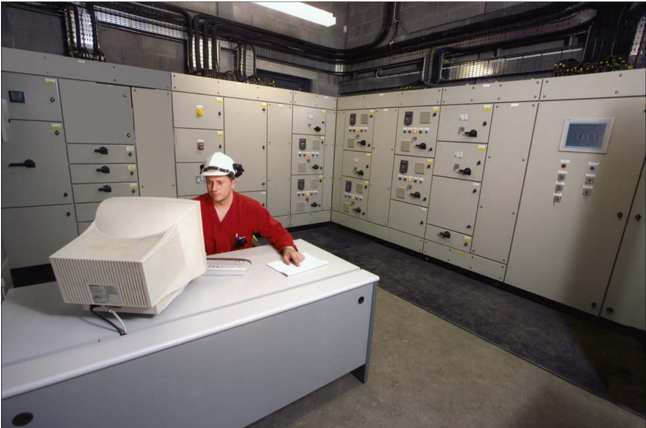
Automation and Process Control Room
